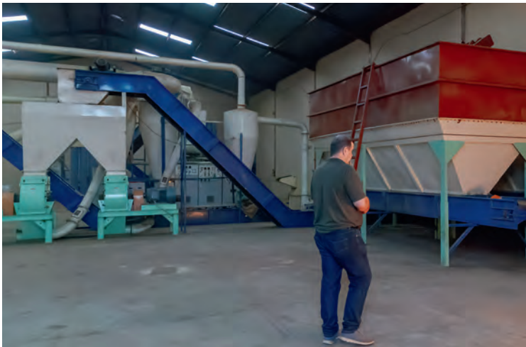
The feedstock receiving hopper and grinders.
