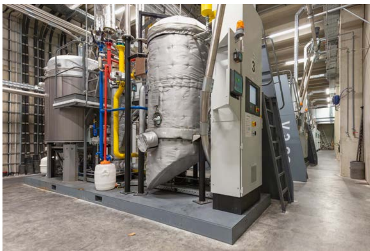
Three Burkhardt V3.90S gasifiers with three CHP ECO 220 units provide 305 kWth and 190 kWe each, consuming c 370 kg of pellets per hour in total.
