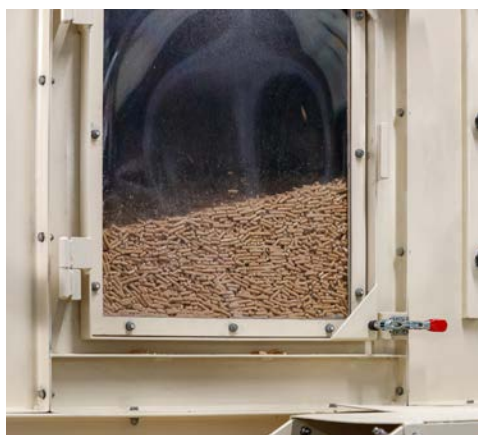
A CPM CounterFlow cooler serves both presses.
