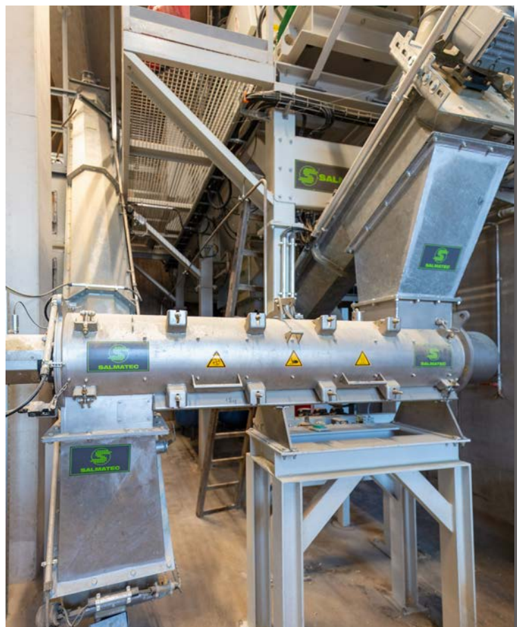
The feedstock preparation, dry grinding, makes the best use of gravity and the compact space.
