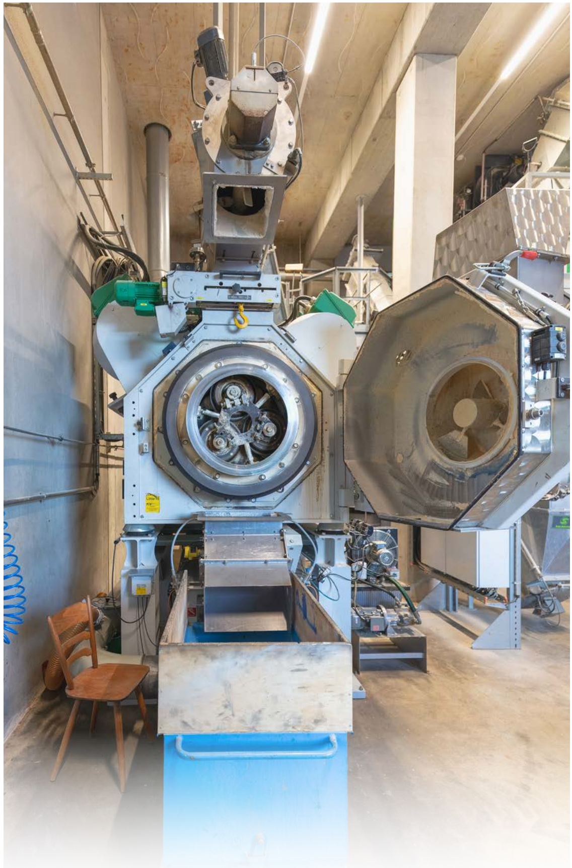
A turnkey delivery by Salmatec, the heart of the Bullinger pellet plant is a single Maxima 700 unit, which according to Salmatec, has a nominal production output of 2 to 3.5 tonnes per hour depending on the material used.
