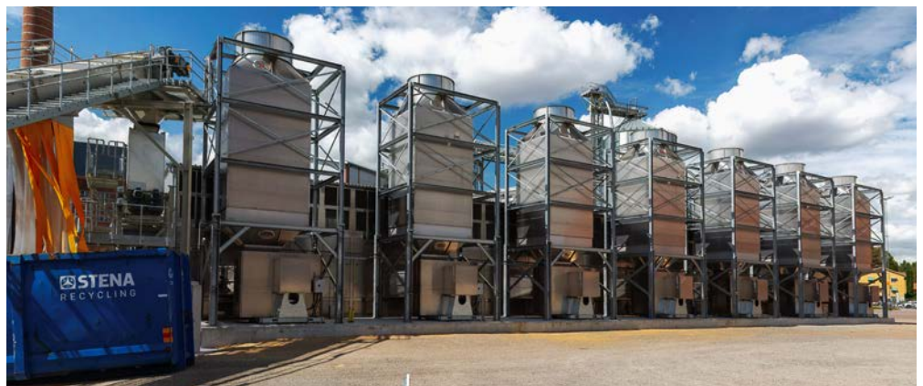
The Stela belt-dryer with the infeed on the top left. The conveyor is fitted with an emergency wastegate.
