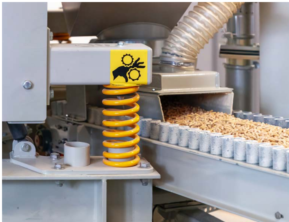
A Mogensen oscillating screener removes fines which are fed to the boiler.
